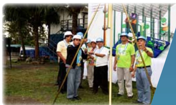
Breaking ground on a biomass cogeneration plant in La Union Province, the Philippines (May 28, 2010)
